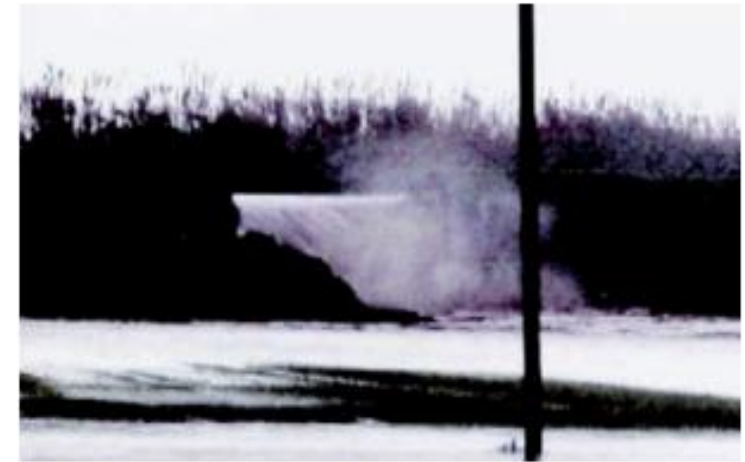
District of Pisa: piping phenomenon through the embankment (landside over the riverbank). From "La voce del Serchio".
